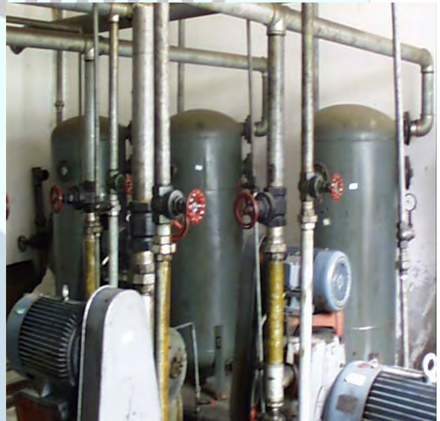
Missing pipe labels.
