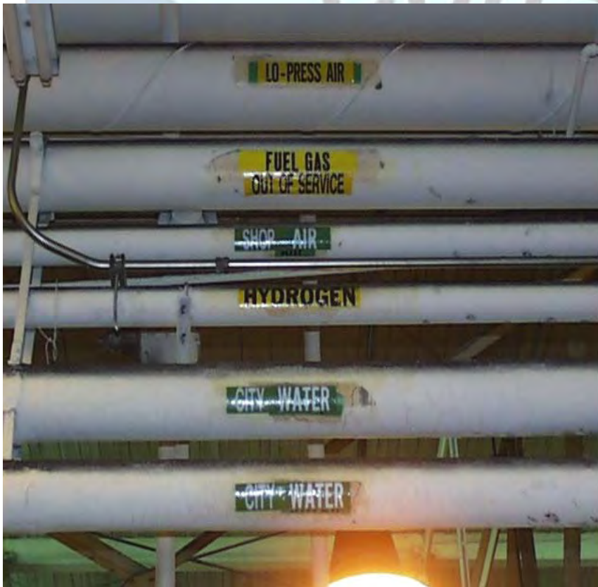
Proper pipe labels.
